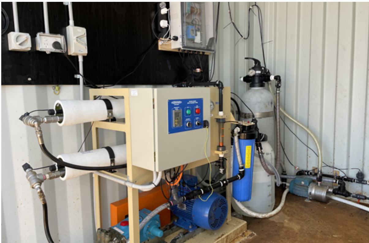
Picture: Prototype reverse osmosis desalination plant operating in Dumbleyung townsite.
